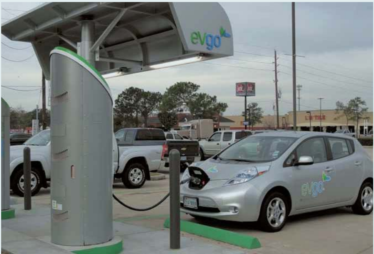
↑ Station de recharge Nissan Houston Texas.
